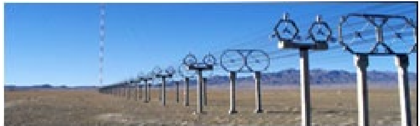
Figure 18: Open feeder line from transmitter to antenna at Dalandsadgab
